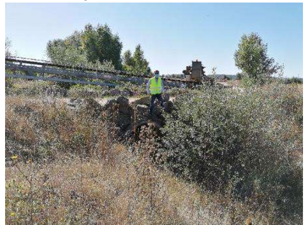
Figure 7: P4 - Exutoire trop-plein bassin A
