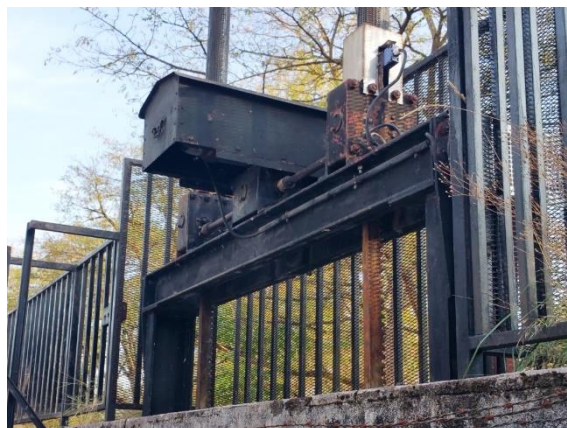
Figure 2-2 : Equipements existants – Vanne murale
