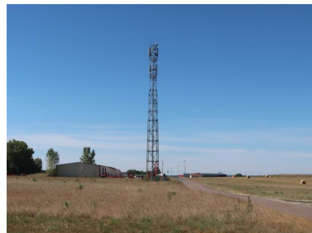
Antenne-relais Source : ARTIFEX 08/2022
