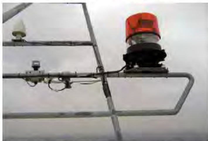
Figure 4. The Vaisala PWD20W installed on a wind turbine in the recommended location below the obstruction light on the nacelle.
